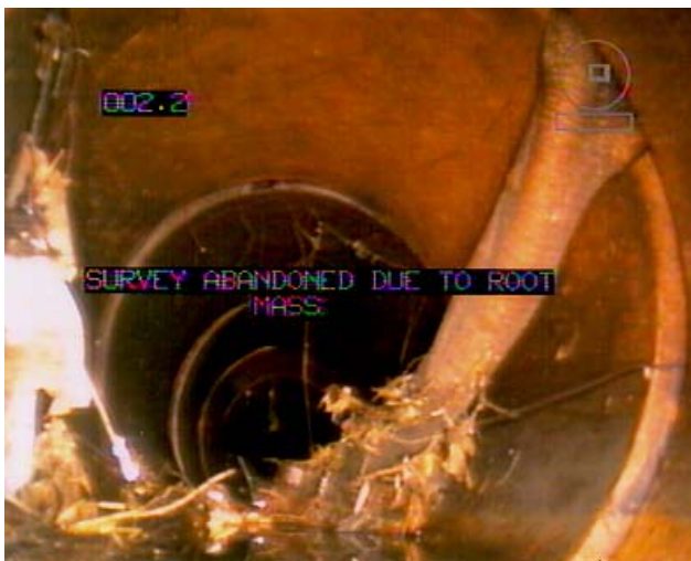
Figure 5: Intrusion into pipe by tree roots pipe
