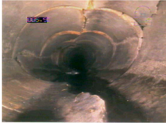
Figure 1: Extremely damaged pipe that still conveys stormwater effectively
